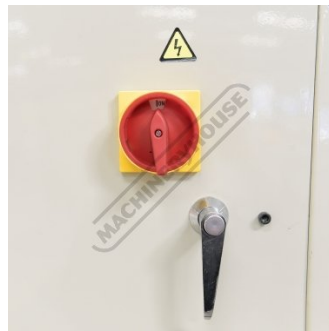
Main Isolation Switch
