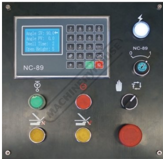
NC 89 Control Panel
