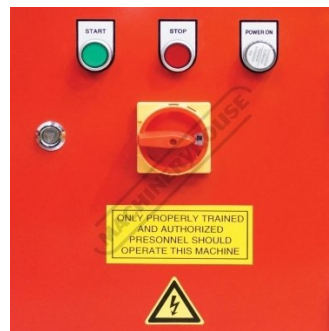
Control Panel Switches
