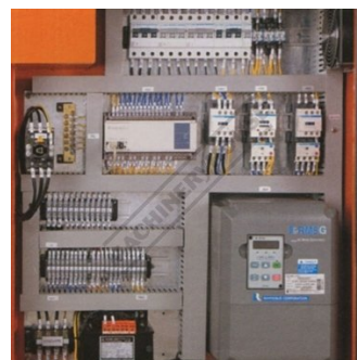
Electrical Control Cabinet
