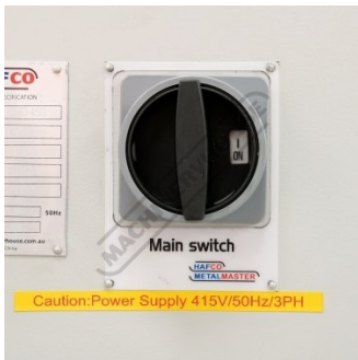
Main Isolation Switch
